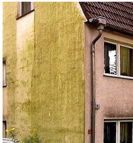
Abb. 13: extremer Algenbefall (bau-praxis-blog, 2011)
